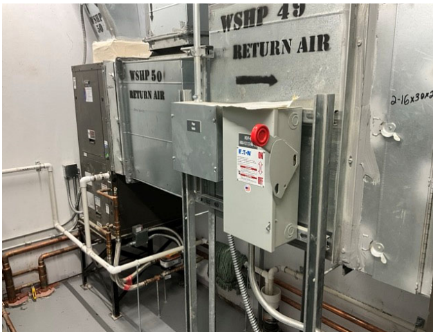
27 - SECONDARY MECHANICAL ROOM
