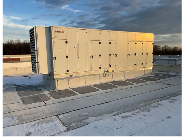
26 - ROOFTOP MECHANICAL EQUIPMENT
