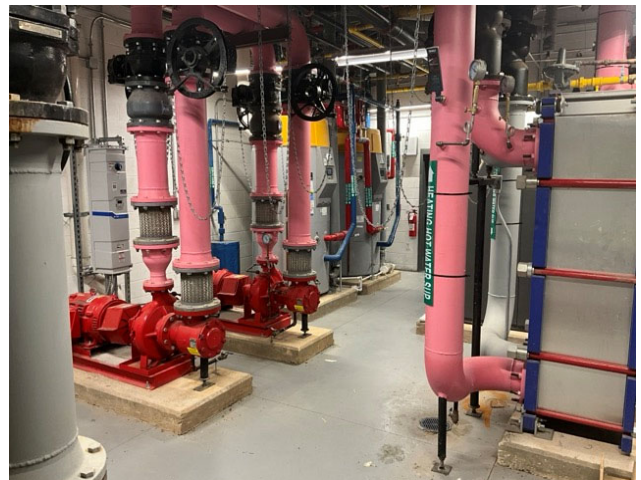
28 - MAIN MECHANICAL ROOM
