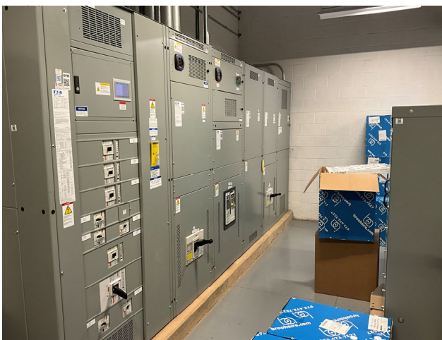
29 - MAIN ELECTRICAL ROOM
