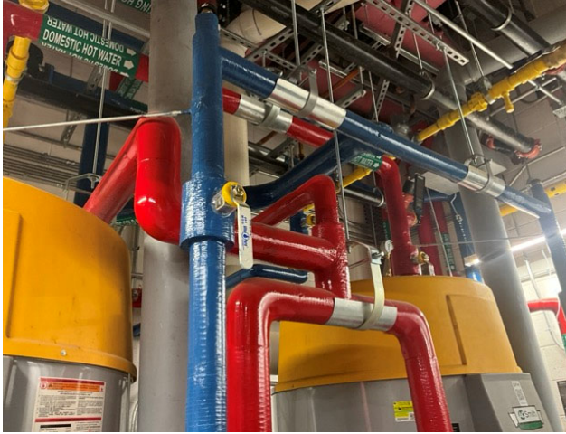
25 - DOMESTIC WATER PIPING
