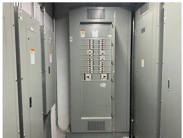
30 - SECONDARY ELECTRICAL ROOM
