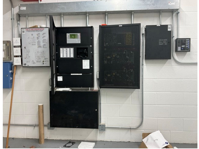
32 - FIRE ALARM PANEL
