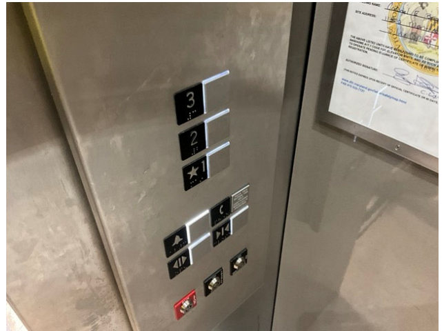
22 - ELEVATOR CAB PANEL
