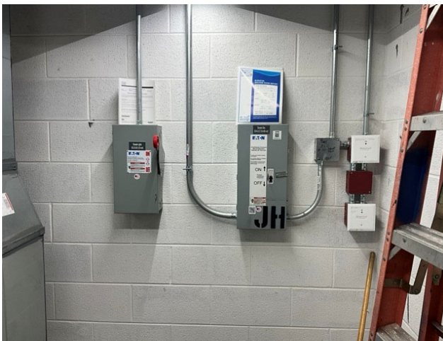
23 - ELEVATOR CONTROL ROOM
